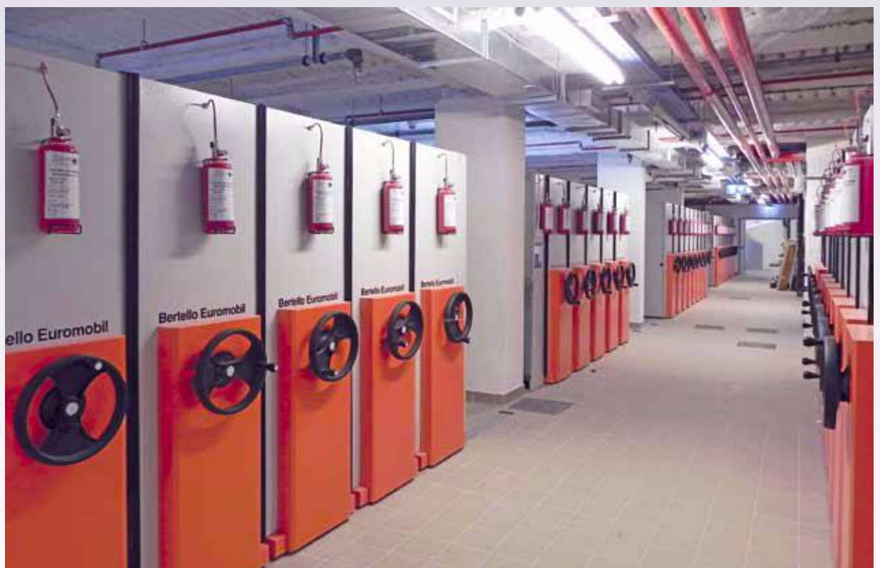
Compact mobile filing system with fire-fighting system
